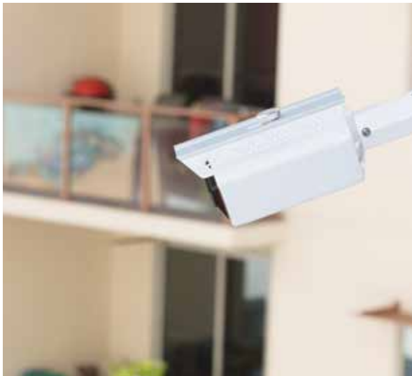
CCTV CAMERA, SWITCHING ON DARWIN PROJECT
