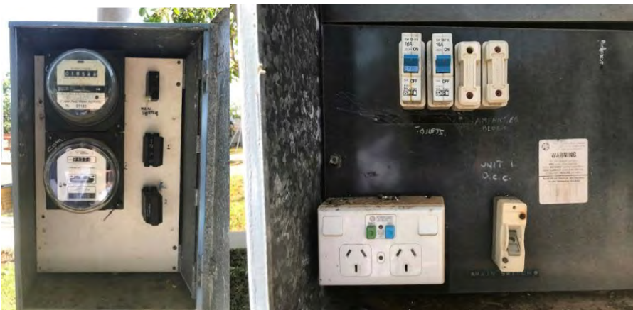
Figure 2 – (L) Metering Panel – Door Open (R) Amenities Switchboard – Door Open
