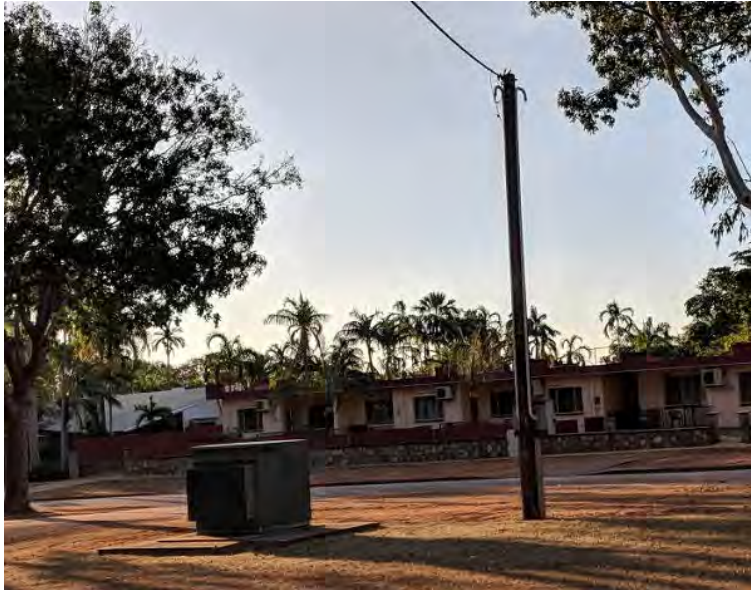
Figure 1 – PWC Substation and Metering Panel
