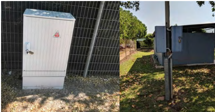
Figure 1 – (L) PWC LV Pillar (R) Pole mounted Meter Panel and Amenities Switchboard
