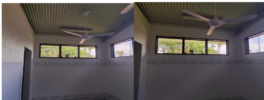
Photos of someone being able to see in from outside whilst standing at ground level
