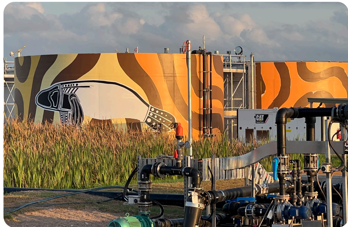
Shoal Bay Leachate Treatment Plant – Artwork Brolga and Dugong by Trent and Jason Lee 2022
