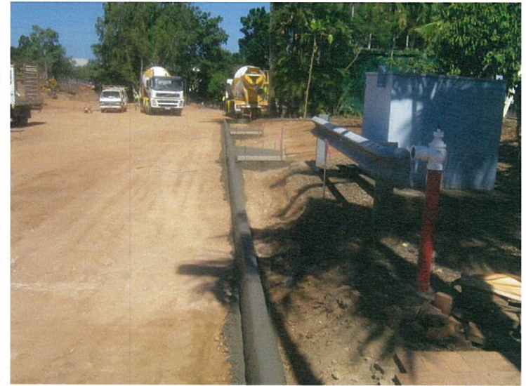
Northern Territory Fire & Rescue Services Car Park
